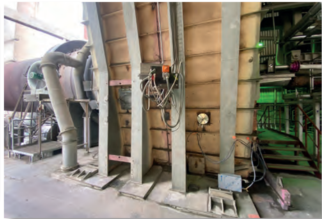
Figure 9: View of the receiver at the kiln hood
