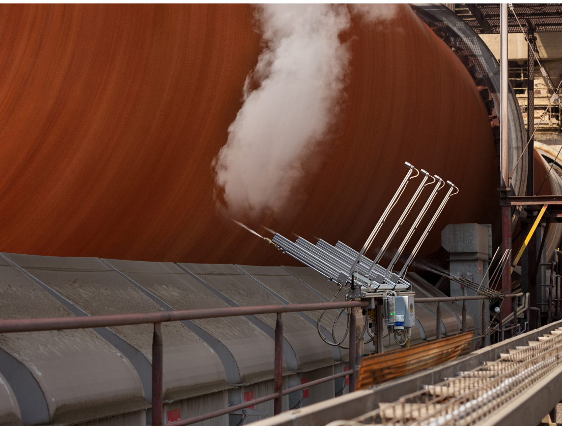
KilnCooler Hot Spot – in action
