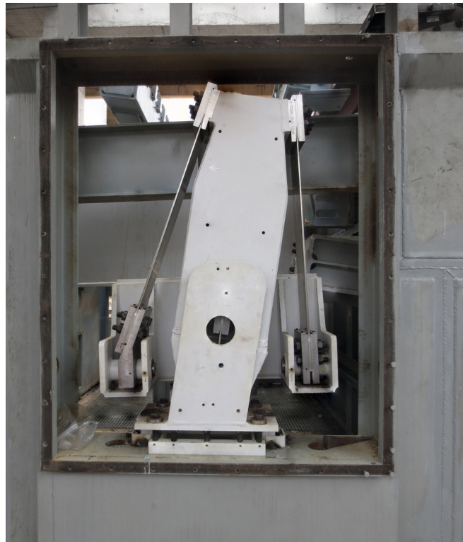
LPS® installed in cooler housing
