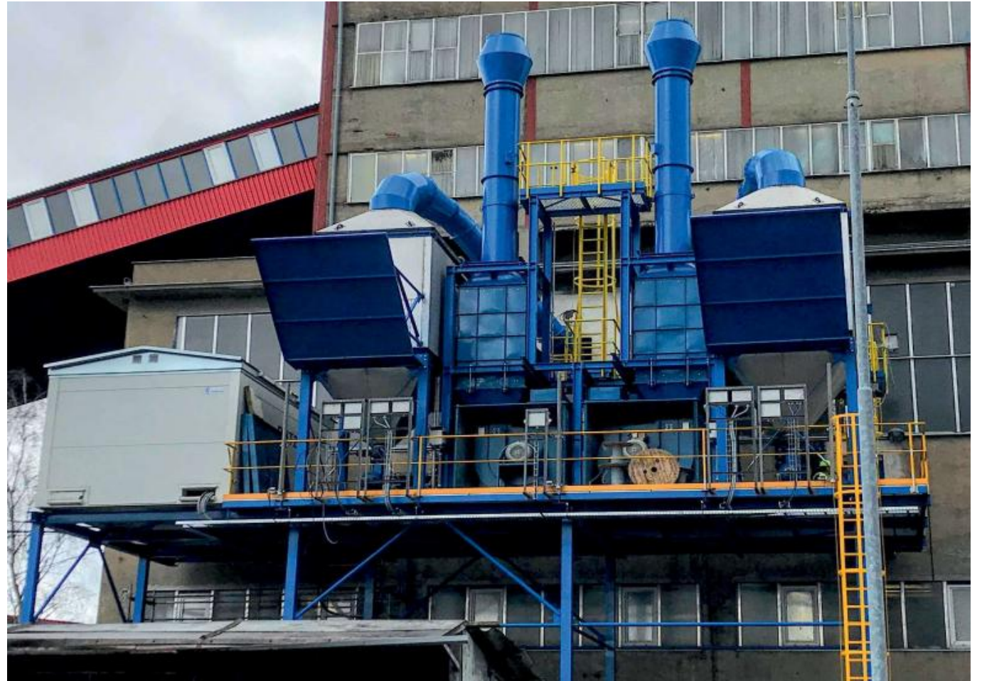
Screening plant dedusting
