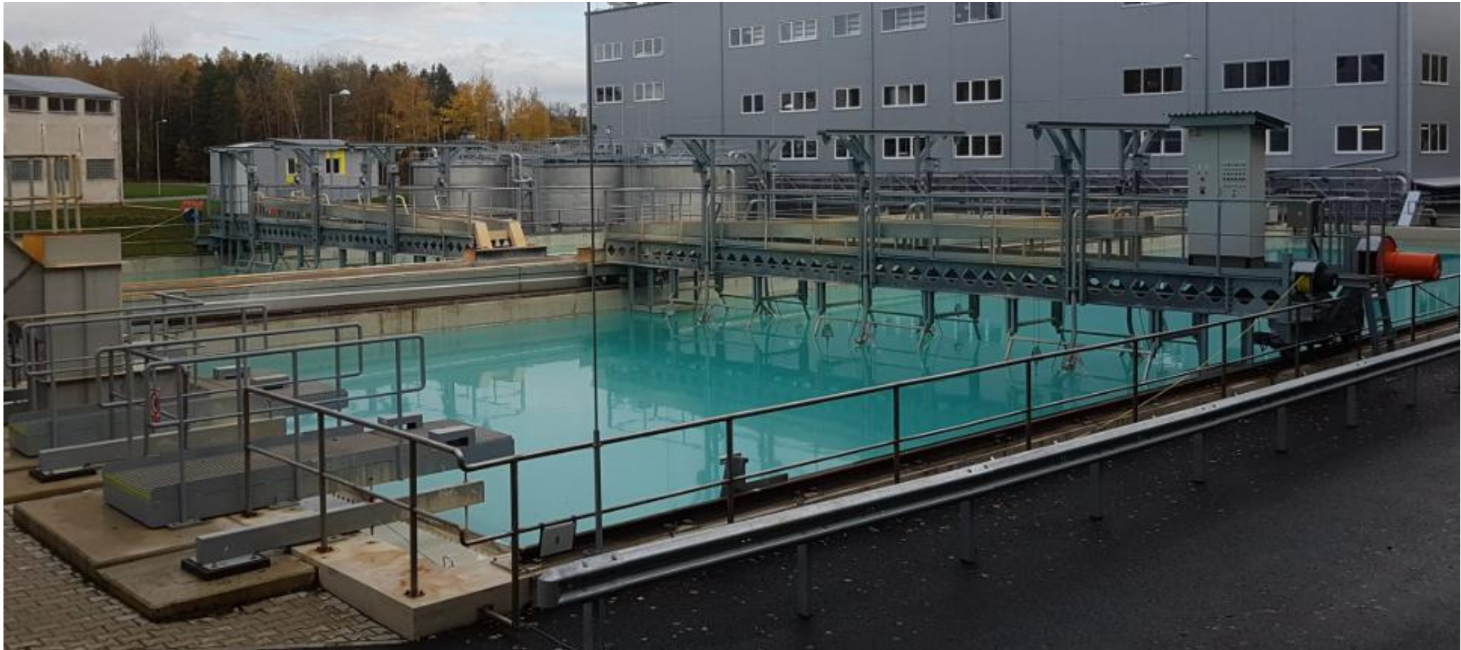
Revamping of neutralization and decontamination station
